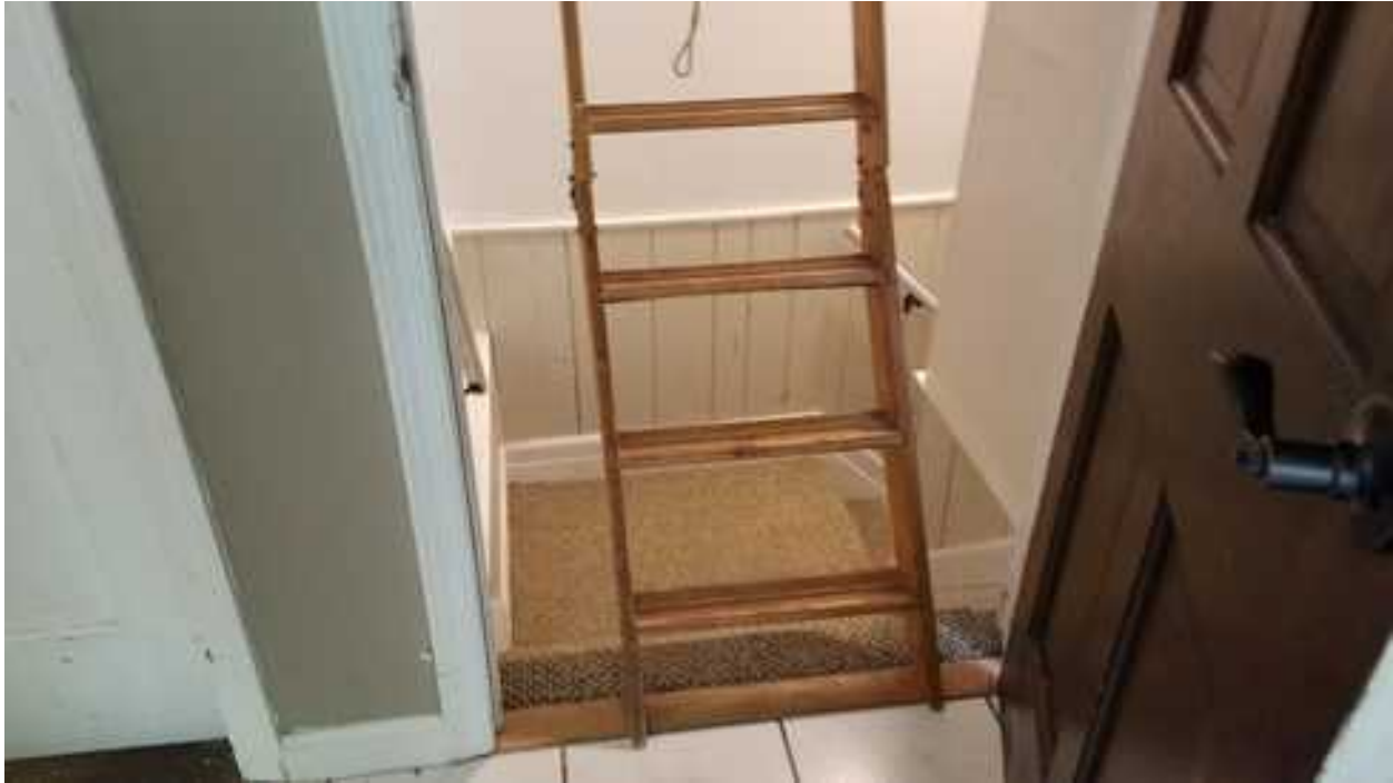
7C.03 Window, bedroom: less than 4-sq. ft. operable, too high off floor etc. in the basement (egress concern). Repair is recommended. This is a safety concern. This is an expense concern
