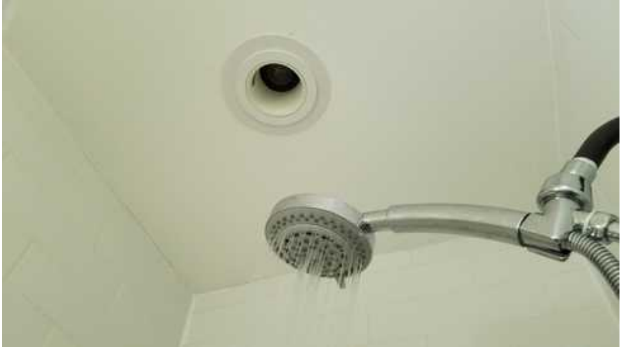
Recessed lighting does not appear to be IC rated (chrome finish not present) for material contact in the attic. Repair/replacement is recommended. This is a safety concern
